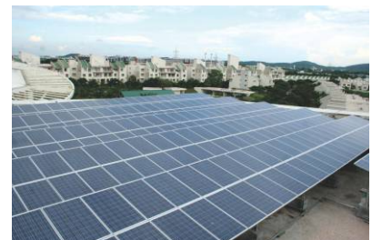
Rooftop solar PV at 'Evolve' MWC, Jaipur
