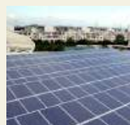
75 Kw Rooftop Solar system installed at MWC, Chennai
